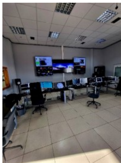
Figure 6 The Control Room at GRANTECAN
